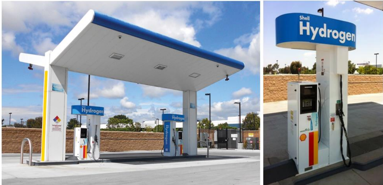
Figure 20 Shell Hydrogen Fueling Station
