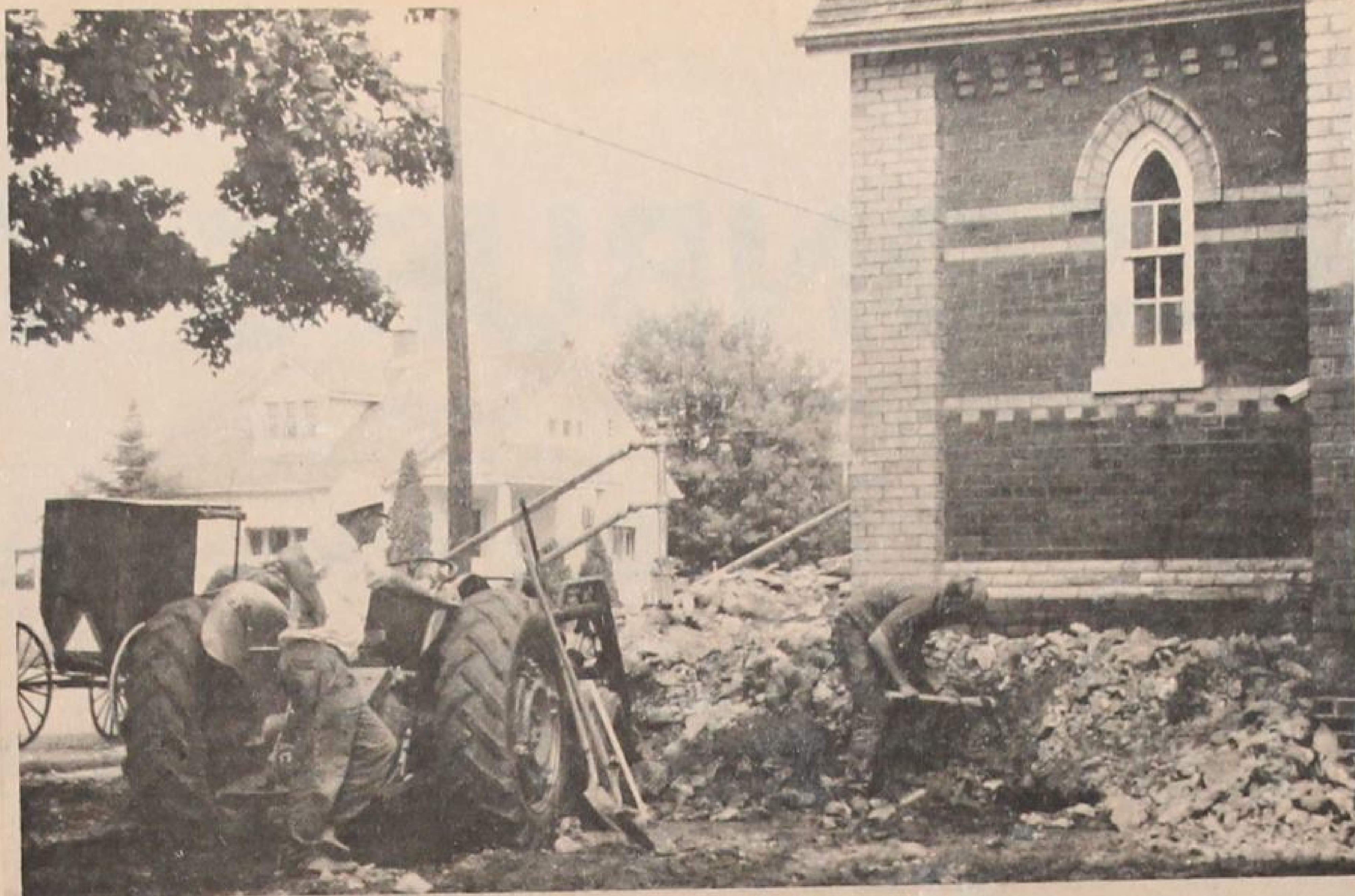
The United Church of Springford is getting a new front step, but the old one isn't giving up without a struggle. Although grass was growing through the old sidewalk, workmen discovered to their chagrin that it is two feet thick! Savili Construction, Otterville, is doing the work which will be completed this week.
