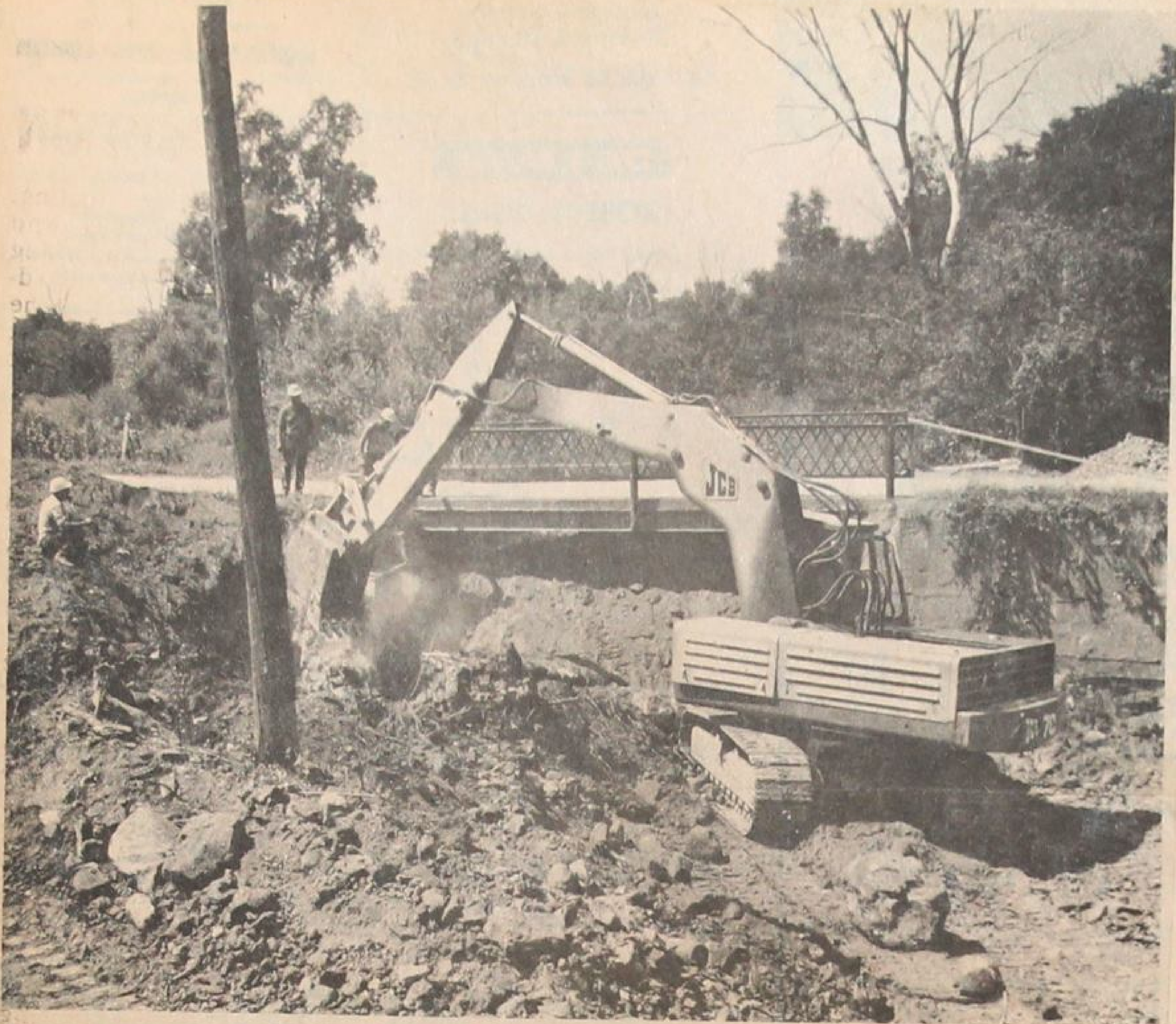
Construction has begun on the Branch Creek Bridge on the road between lots 11 and 12, Concession 8, South Norwich. Facca Construction Company, Windsor, is building the reinforced concrete structure, which will be 35 feet by 16.95 feet by 24 feet. The tender price is $28,400 and the total cost is estimated at $37,551.90. The old bridge was beginning to weaken at the northern end. The new bridge is being built along side the old.
