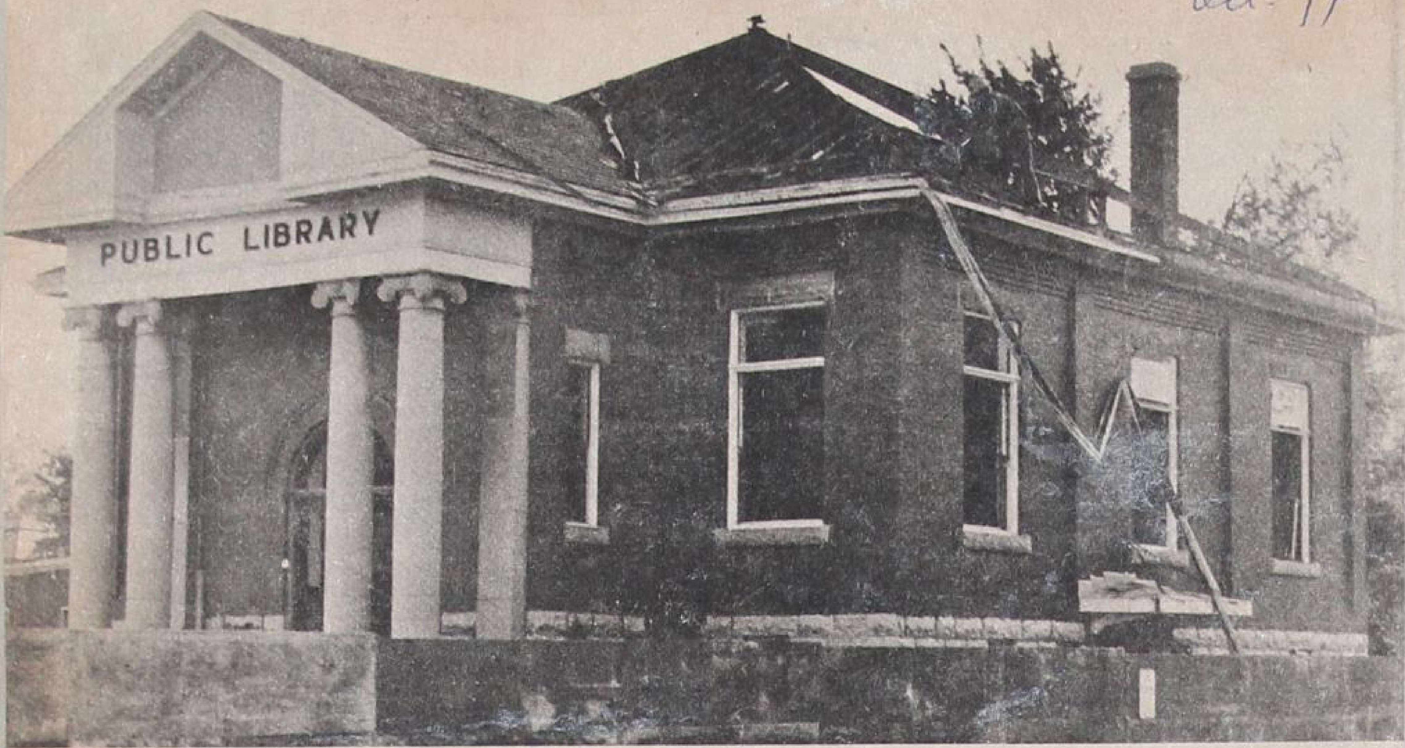
And down it comes. Demolition of the old Tillsonburg Public Library is now well underway, and the building lost its roof sometime yesterday. Demolition of the library, and construction of the new Tillsonburg Public Library on the same site, are being
