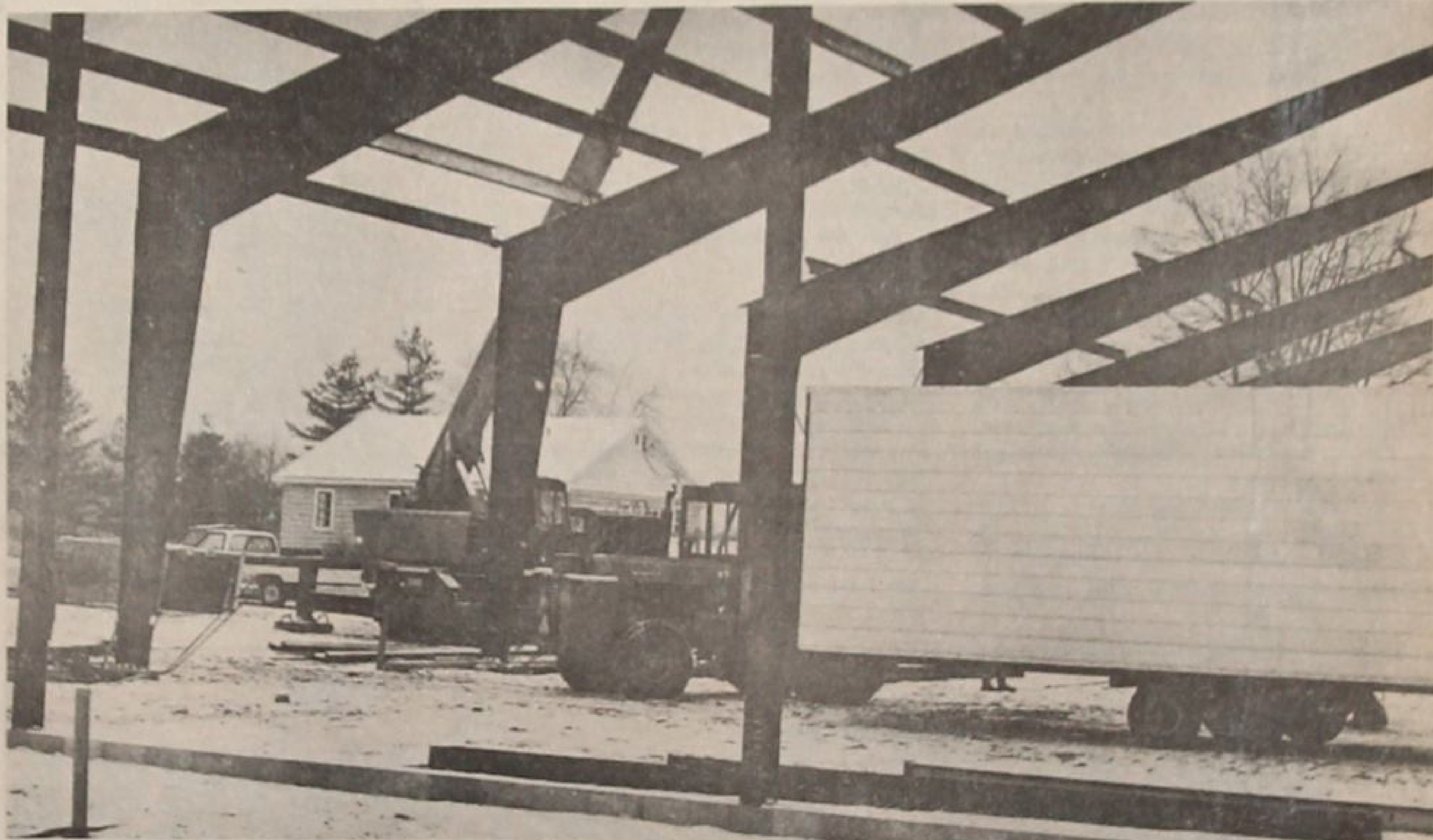
The partially completed Powell Agri-Systems expansion is shown here. The company hopes to have the 15,000-square-foot addition
