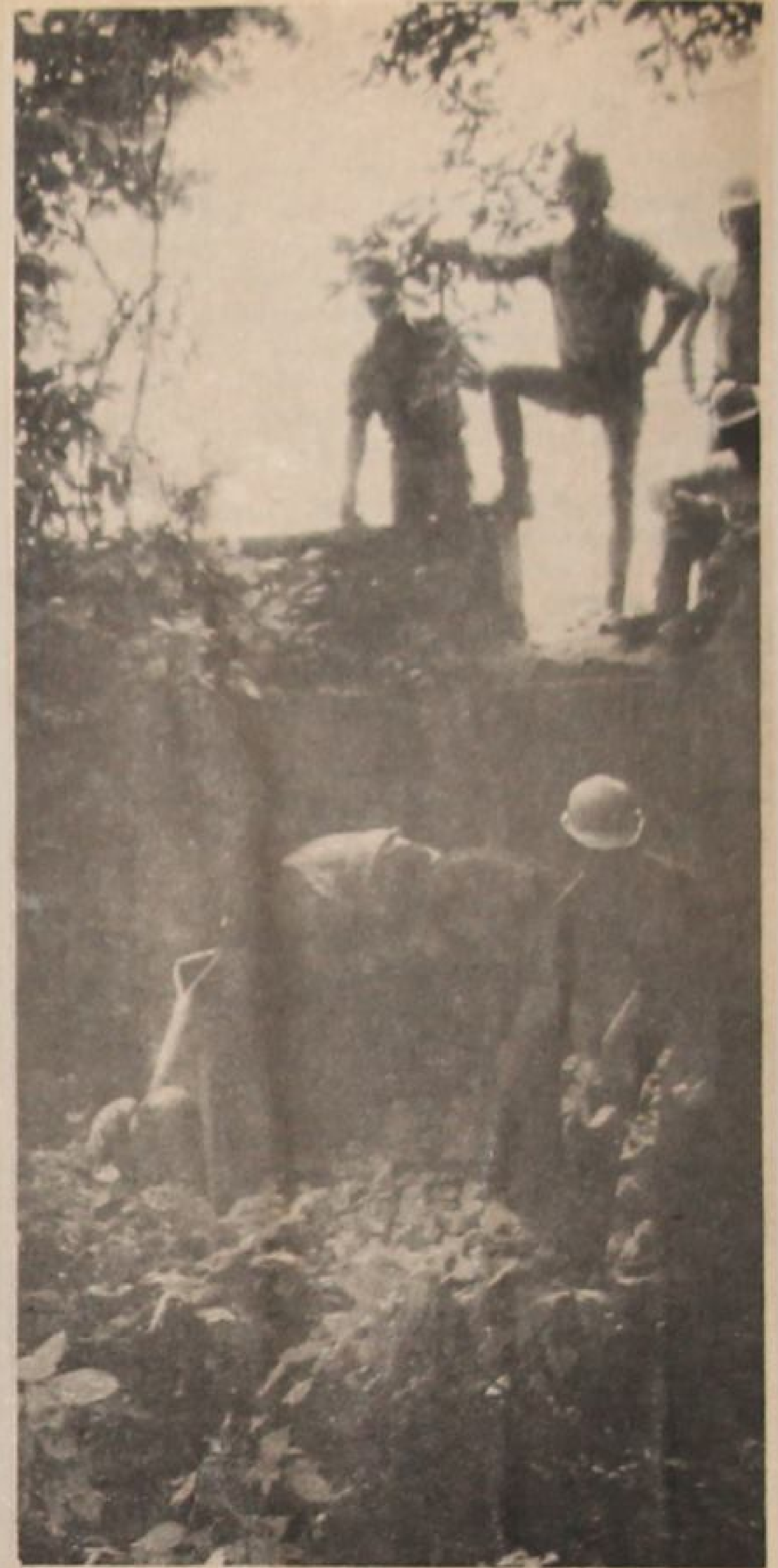
Nine Junior Rangers in co-operation with the Long Point Region Conservation Authority constructed an erosion control structure near Milldale recently. At the request of land owner Ken Mann, the team installed 18 tons of crushed rock and gabion baskets. The LPRCA will advise on erosion problems of private land owners at their request and will split the cost of some erosion control projects.
