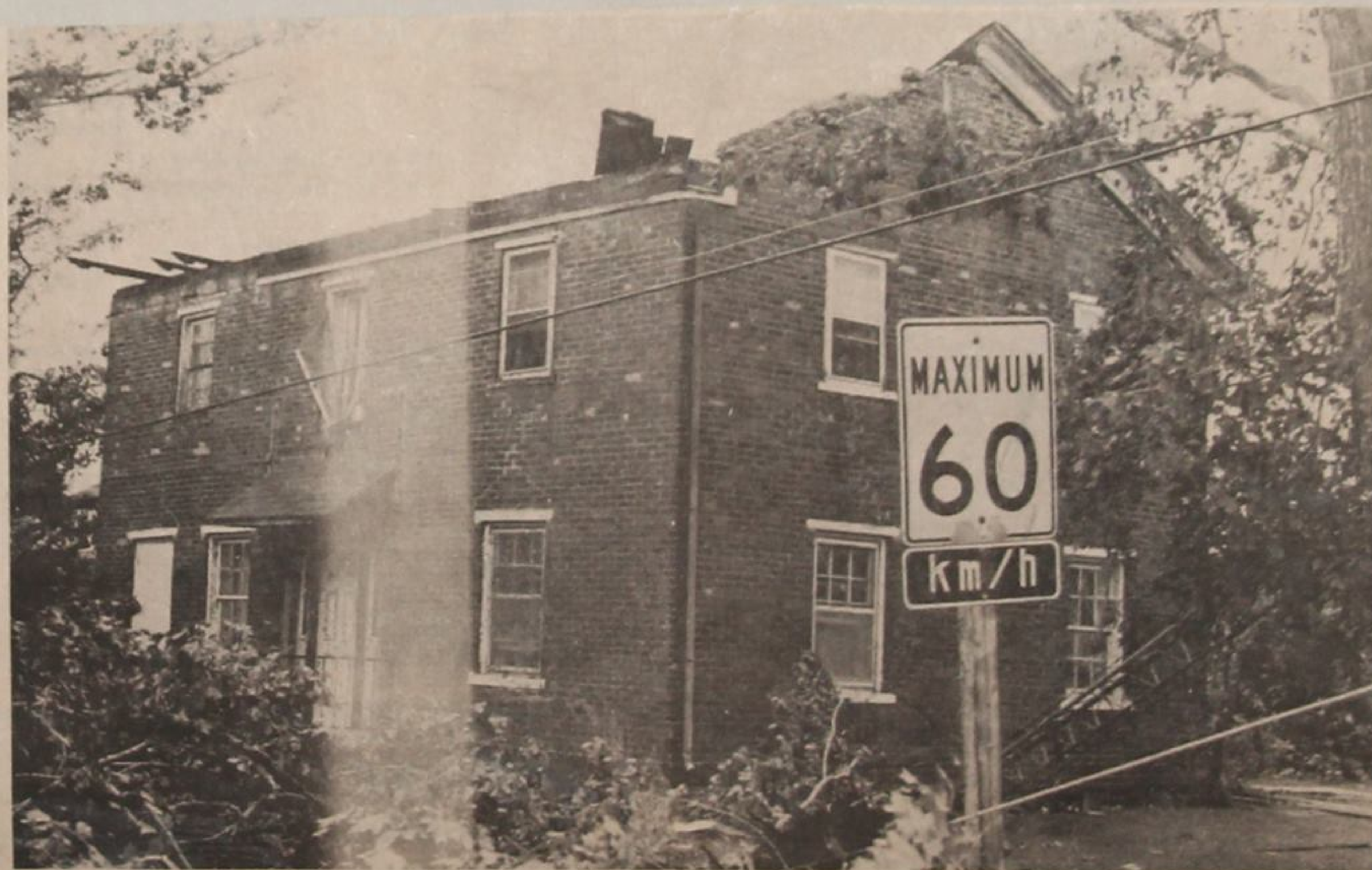
Last night's tornado paid no heed to this speed limit sign in front of this New Durham house.
