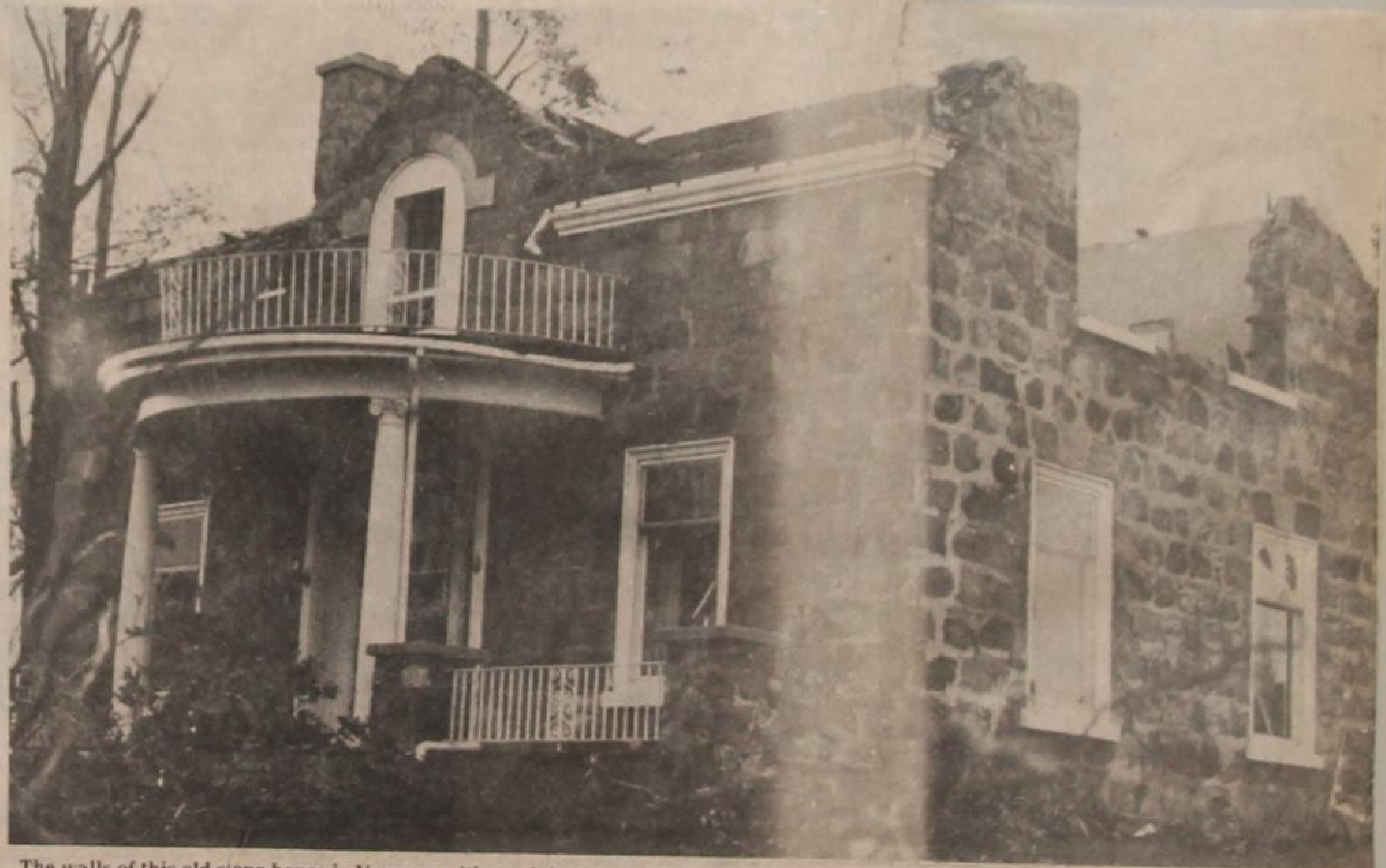
The walls of this old stone house in Vanessa withstood the force of Tuesday's tornado, but the roof did not.
